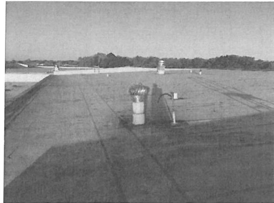
View looking west from the rooftop. Venting system wind turbine located in center of photo.
