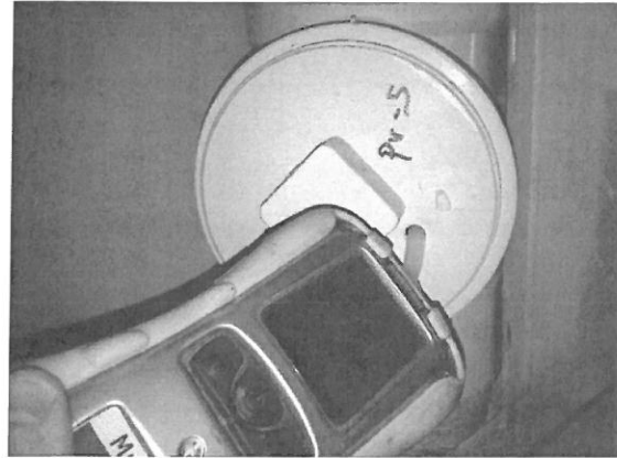
View of measuring for methane and LEL at the V-5 riser pipe for the passive venting system.
