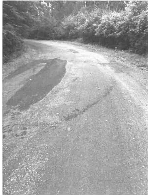
Figure 11: 103 rd Street N – showing patching, roadway potholes, deteriorating pavement
