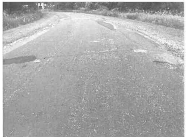
Figure 12: Greenlefe Avenue N– showing roadway potholes, multiple patching & failing bituminous edges
