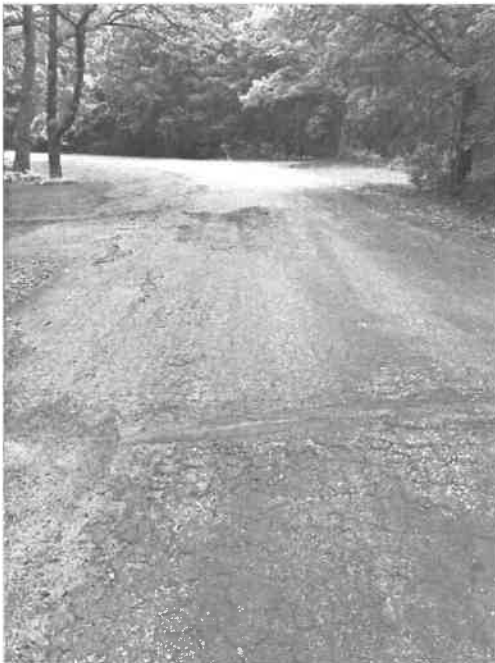
Figure 2: Janero Court N - showing alligator cracking and failed bituminous
