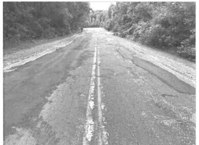
Figure 4: Joliet Avenue N – showing major spot patching and pavement deterioration
