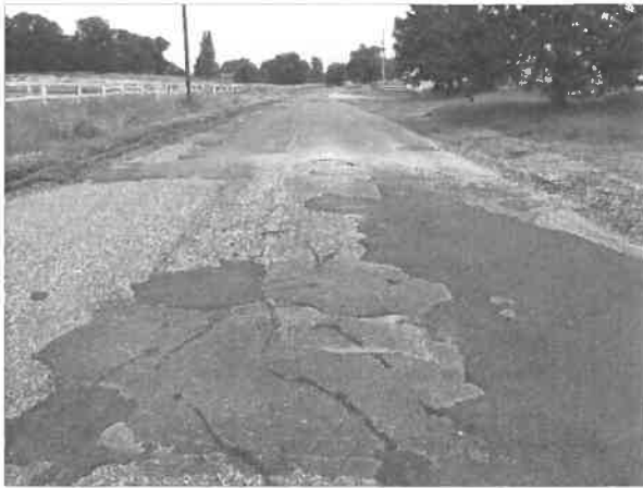
Figure 1: Justen Trail N –showing signs of serious pavement distress including multiple attempts to patch
