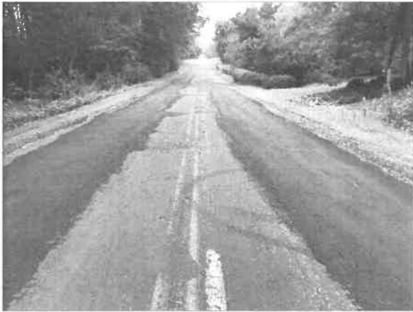
Figure 5: Joliet Avenue N – showing major attempts at road patching
