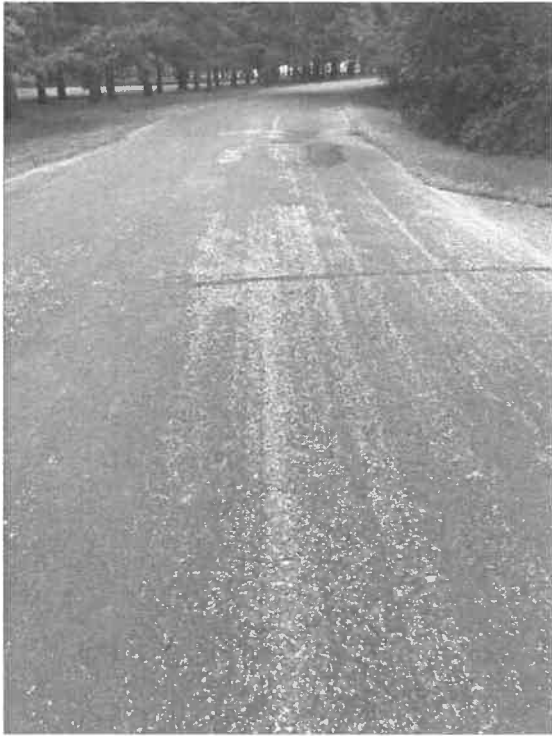
Figure 9: Kelman Court N – showing horizontal cracking
