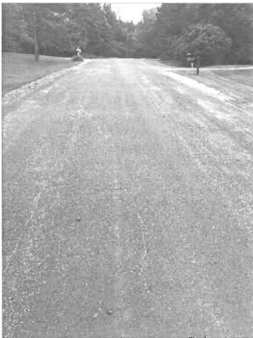
Figure 10: 103 rd Street Ct N - showing pavement distresses including longitudinal cracking & alligator cracking
