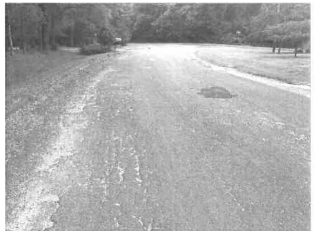
Figure 8: 103 rd Street N– showing crumbling bituminous curb, pothole patching & deteriorating pavement
