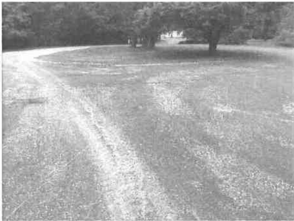
Figure 6: Jody Avenue Ct N - showing longitudinal cracking
