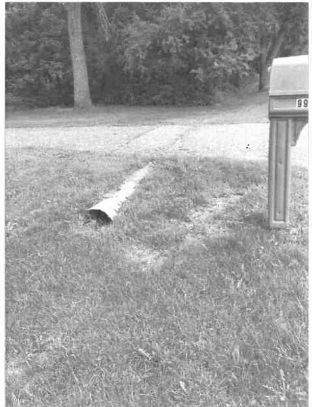
Figure 3: Justen Trail – Driveway culvert in need of replacing
